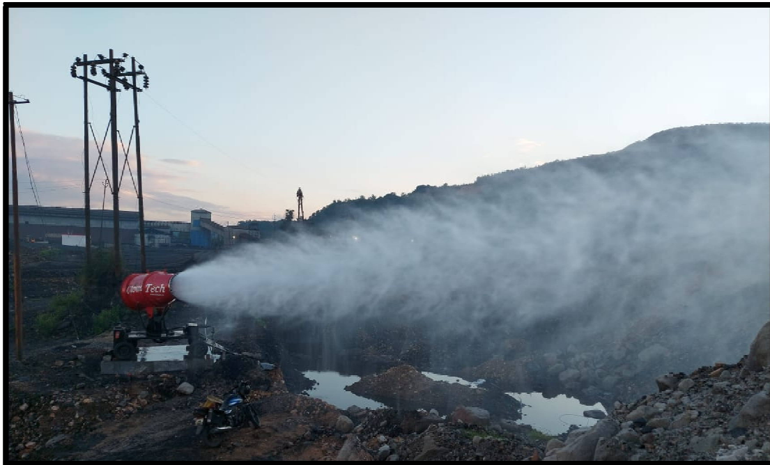
Fixed Fog Canon at Coal yard
