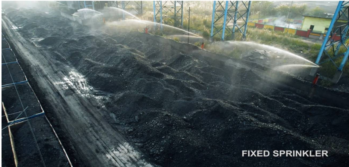
Fixed Sprinklers at Wharfwall
