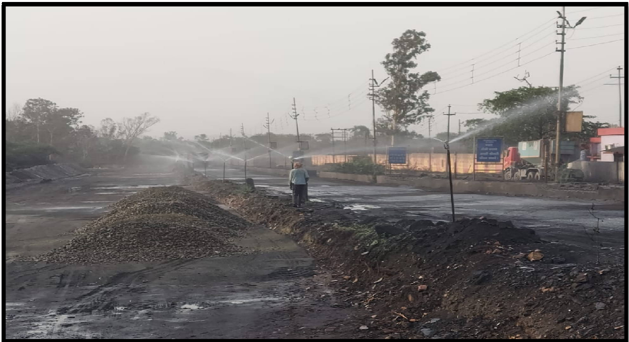
Fixed Sprinklers along RCC approach road
