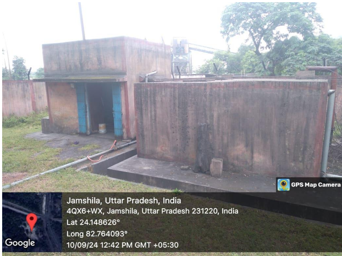
2 no. of Pump house along with storage tank of 0.5 Lakh Litre at Deshaling Plant (within 100 m of deshaling reject yard).
